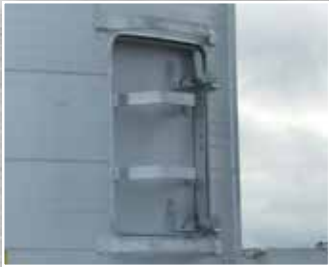
Access Door in Front on Roadside
